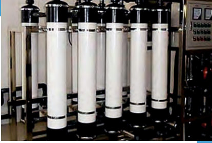
Ultraviolet Filtration Plant
